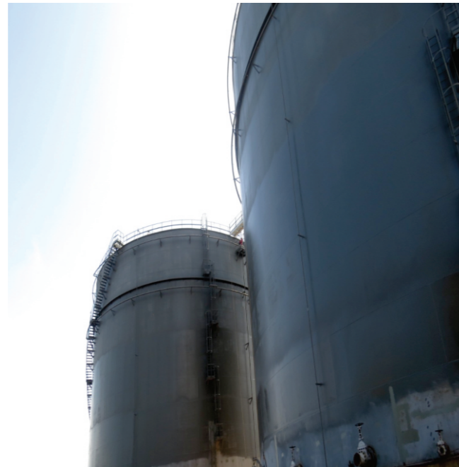
CORNEX (SL) LIMITED TANKS
